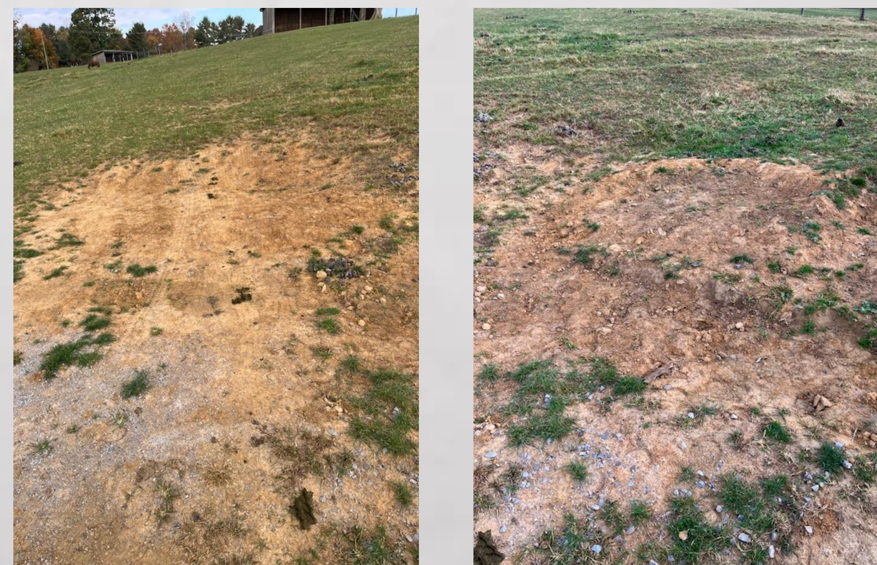
These two images show the installation site after 2 weeks of varied weather. The drain is concealed and the water drains away from the gate
